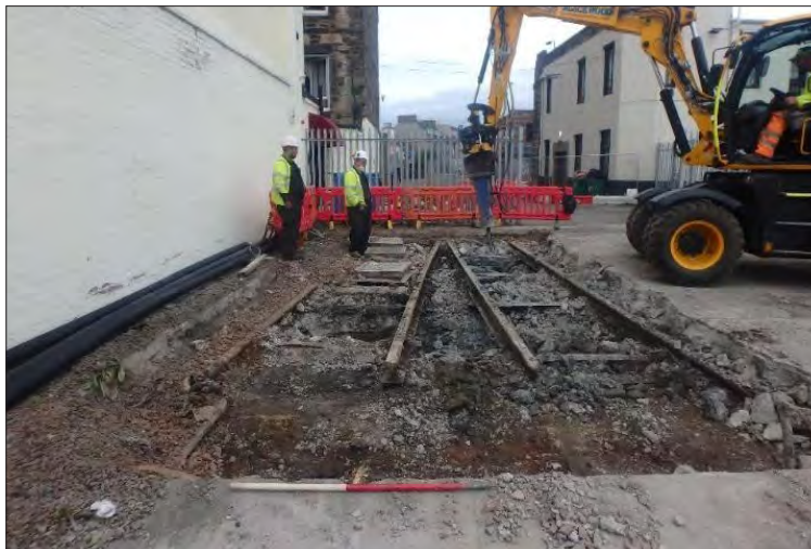
Plate 40: Removing the concrete floor of the bus station to reveal the old tram tracks encased in concrete
