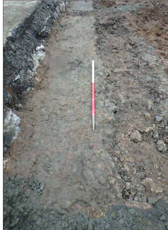
Plate 16: View of the metallated road surface (6903) at the junction of Dalmeny Street (Area 55 and 69)
