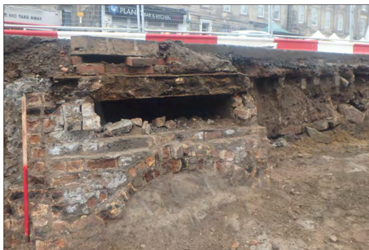
Plate 28: entrance to the corridor running north-west/south-east with arched roof partly filled by foam concrete
