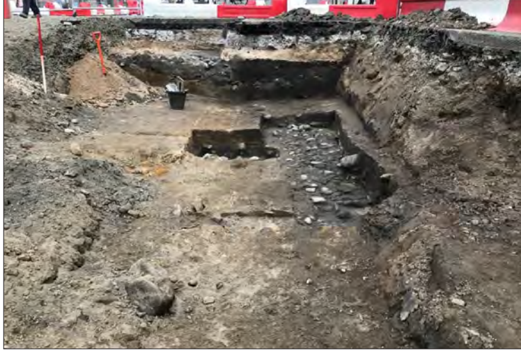
Plate 6: The stone foundation was removed to reveal a cobbled surface (6046) below, from the south
