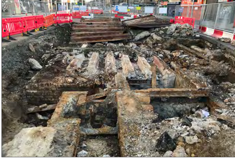
Plate 32: Removing the metal sheet pile roof of the cable house (5705) at Albert Place
