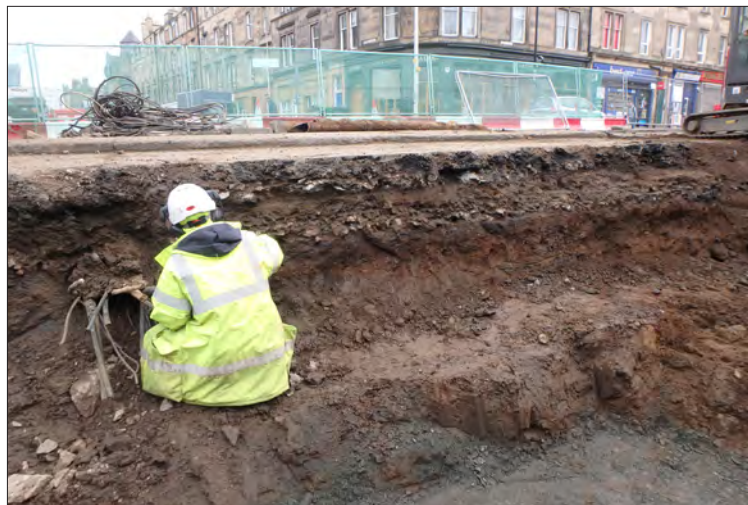
Plate 17: Area 55 and 69, recording the section through the road surface (6903) at the junction of Dalmeny Street
