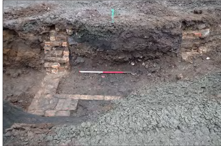
Plate 29: Remains of cables tunnel (7308) discovered in section at south of the rail
