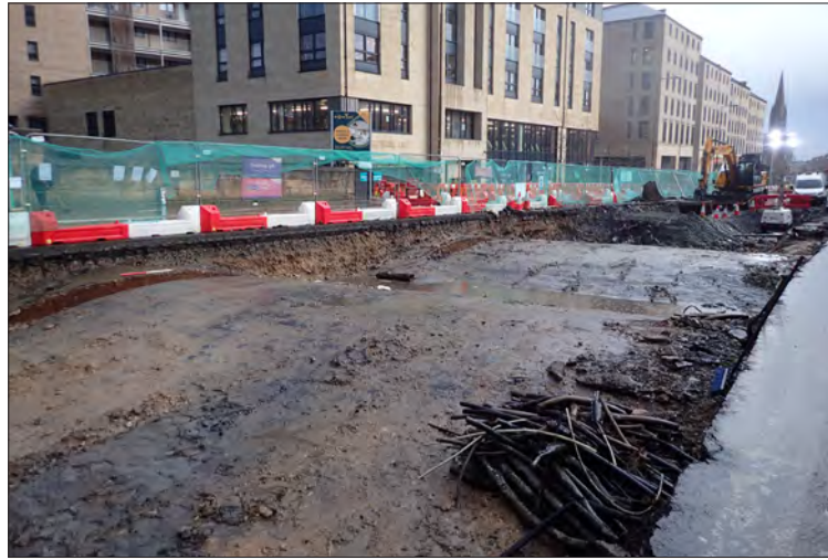
Plate 44: Top of the rail bridge arches exposed during the bulk excavation in area 73
