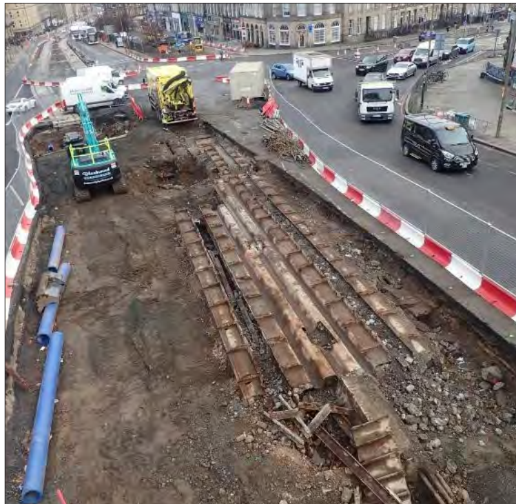
Plate 18: Overhead view of main chamber and cable tunnels at Antigua Street/Baxter's Place
