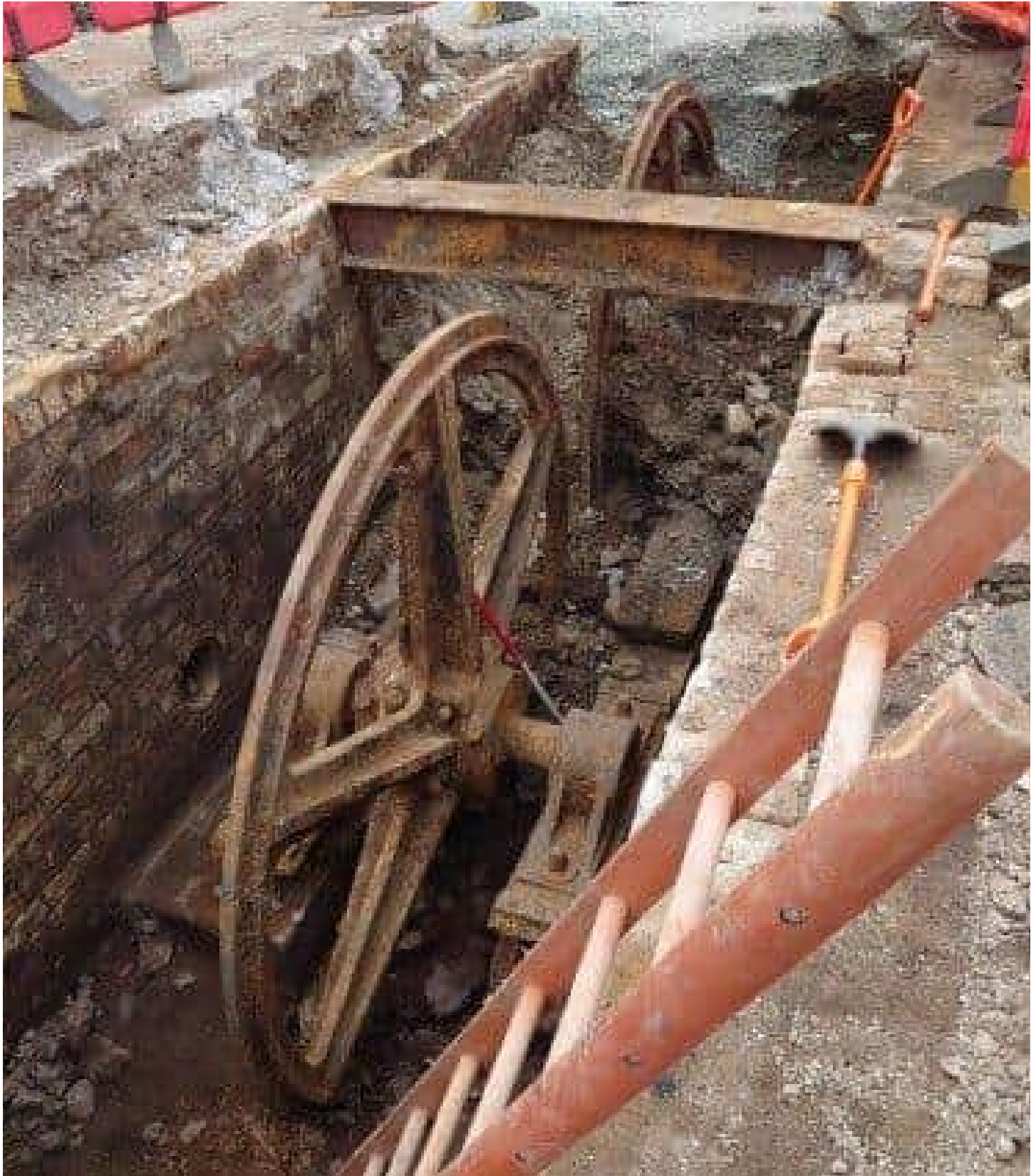
The giant wheels once turned the cables used to power the city's tram network and were rediscovered as work progressed on the new tram network. PIC: Contributed.
