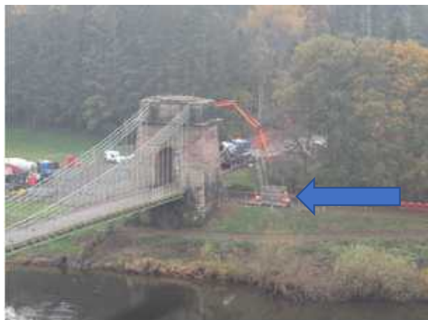
Left: Filling a concrete drum, arrowed, on the English side, which will be used as an anchor for BT cables from beneath the Bridge, relocated for the duration of the works. And below, later in the day, a similar operation on the Scottish side.
