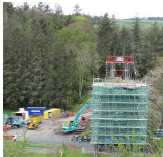
The Scottish tower shrouded in scaffolding, with piledriving machine (blue) to the left – 12 th May
