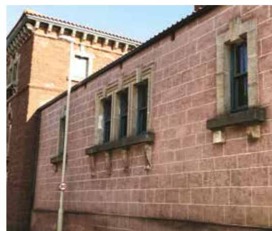
The former boiler and engine house as seen from the road. Even the boiler house had ornate window frames.
